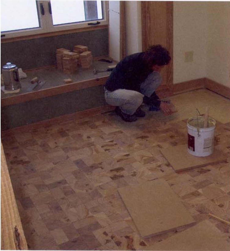
The Parkville couple was intent on creating the smallest amount of waste from their home construction. Here, Kelly Parker installs an end-block floor made from scrap lumber.
